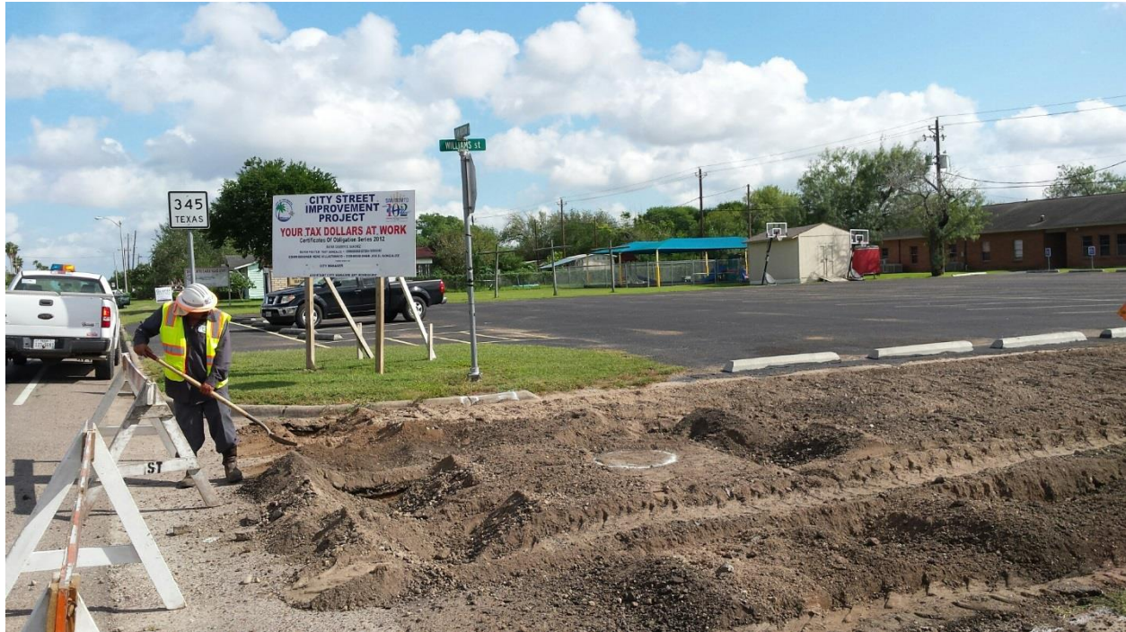
Street Maintenance Crew started working on the Intersection of N. Sam Houston (345) and 3 blocks of Williams Street
